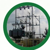
EB & WATER LINE
